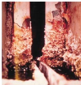
Exterior Corrosion on Metal
