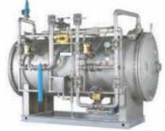
Ozone generation chamber, Instrument & valves
